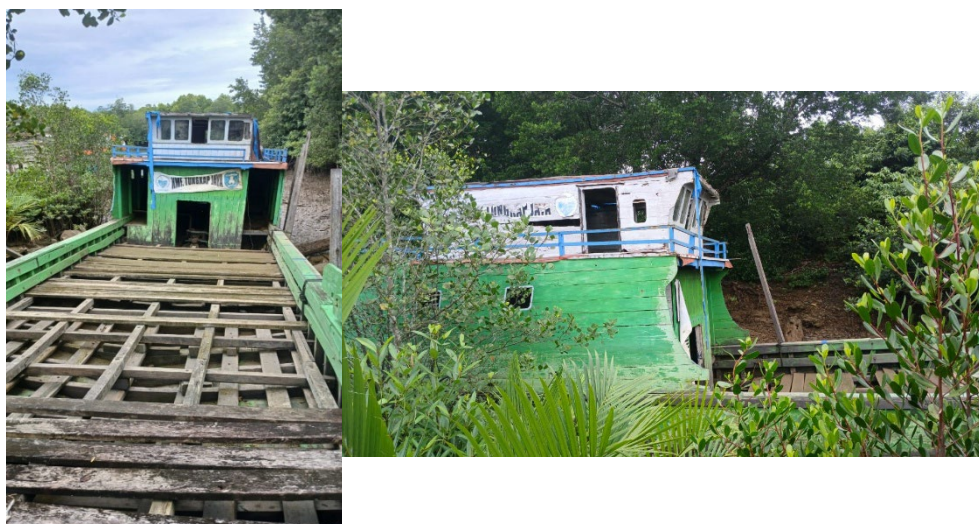
Figure 2. Condition of the Tungkap Jaya BUMDes Ferry, which is Damaged and Out of Service (2023–2025)
